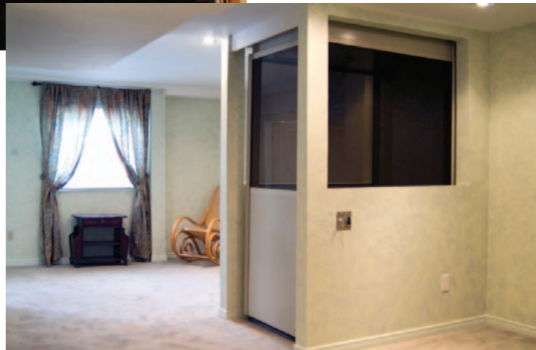
Barrier free residential two storey Telecab elevator installed by ReliAble Living provides complete access for the disabled parents of the home owners.
