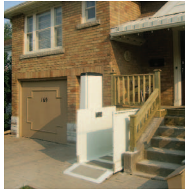
Wheelchair lift installed by ReliAble Living provides the home owners with wheel chair access into their home.
